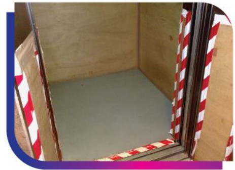
◎ 升降機保護木夾板鋪放困難及不美觀 Lift car protecting wooden board was not user-friendly and unpleasant.
