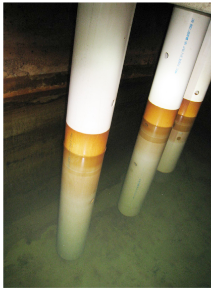
PVC筒導管 PVC ducts
