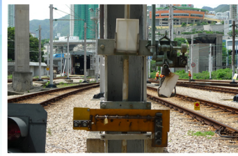
架空天纜的開關系統加裝接地纜聯鎖 The New Castell-Interlock was integrated into OHL Mast
